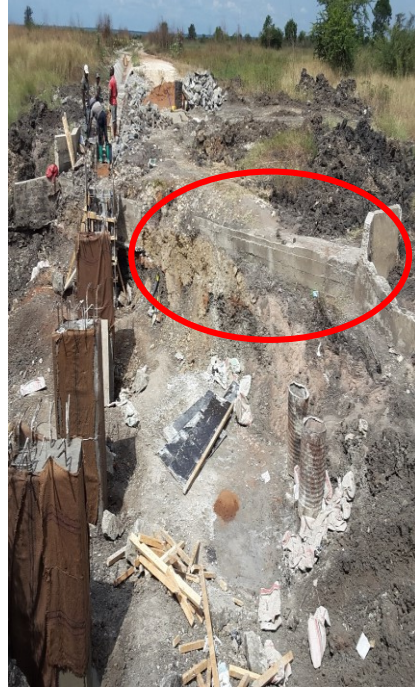
Photo 6.2: Destroyed culvert (Circled red) and construction activities of new structure of aqueduct at Wami-Luhindo Irrigation Scheme. This was due to the impact of skipping aspect of environment on the feasibility study as it was taken by Auditors on 12 th July 2018
