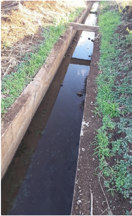
Photo 6.1: Bending inside of Themiya Simba canal due to impact of black cotton soil, taken by auditors on 26 th November 2018
